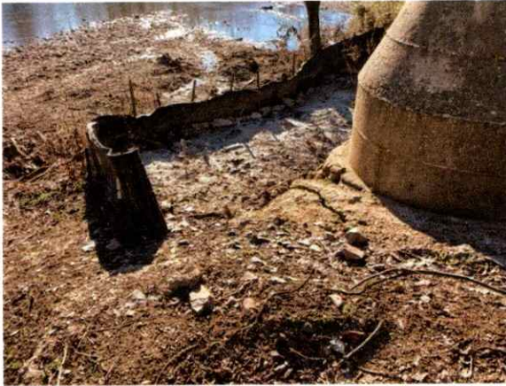
MH 1748 Before Cleanup
